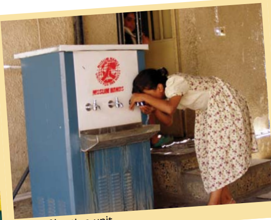
Water filtration unit
